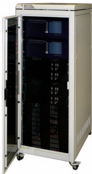
rack mounted panels
